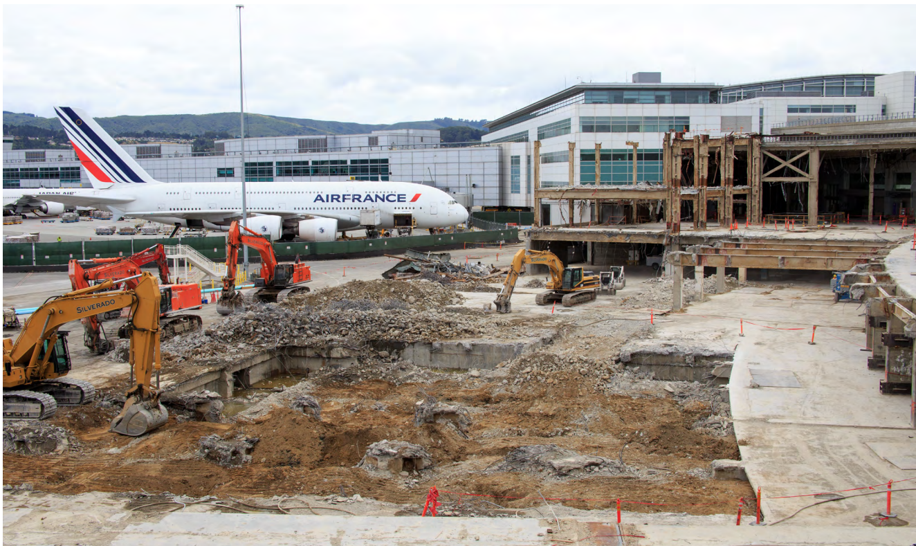
Hensel Phelps executes precise construction adjacent to an active airfield gate, ensuring safety and efficiency during airport operations.
